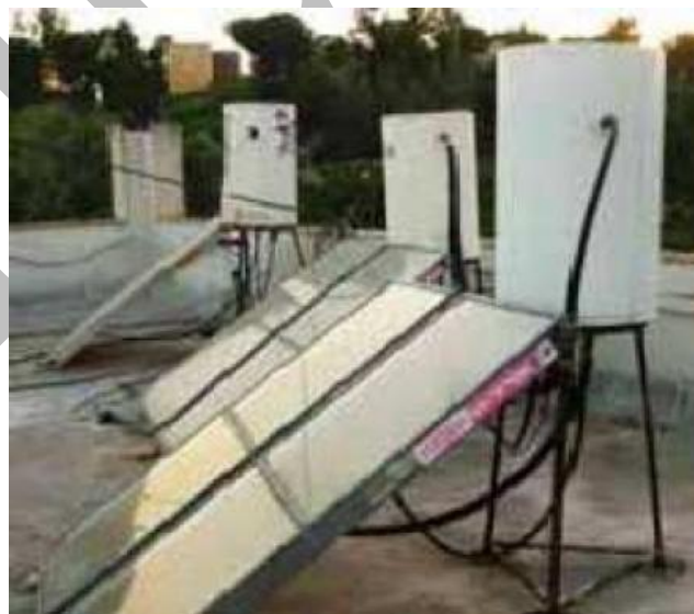
Fig.1. Solar water Heater
